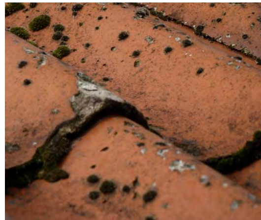
Friable roof surface (4.14)
